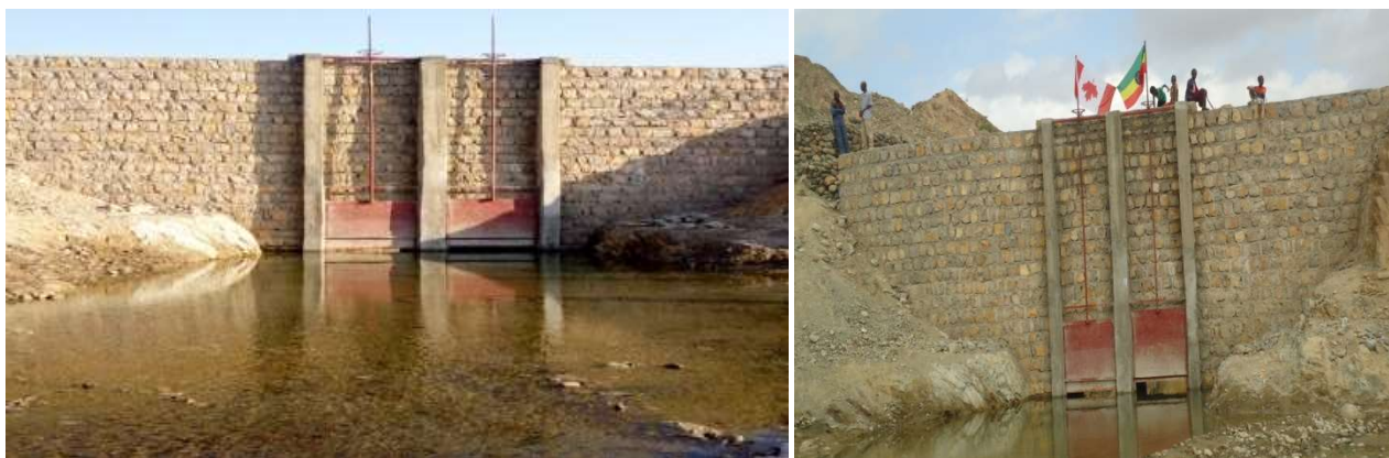
Figure 1: Installed Main canal gate at the retaining wall to control water diversion to the canal
